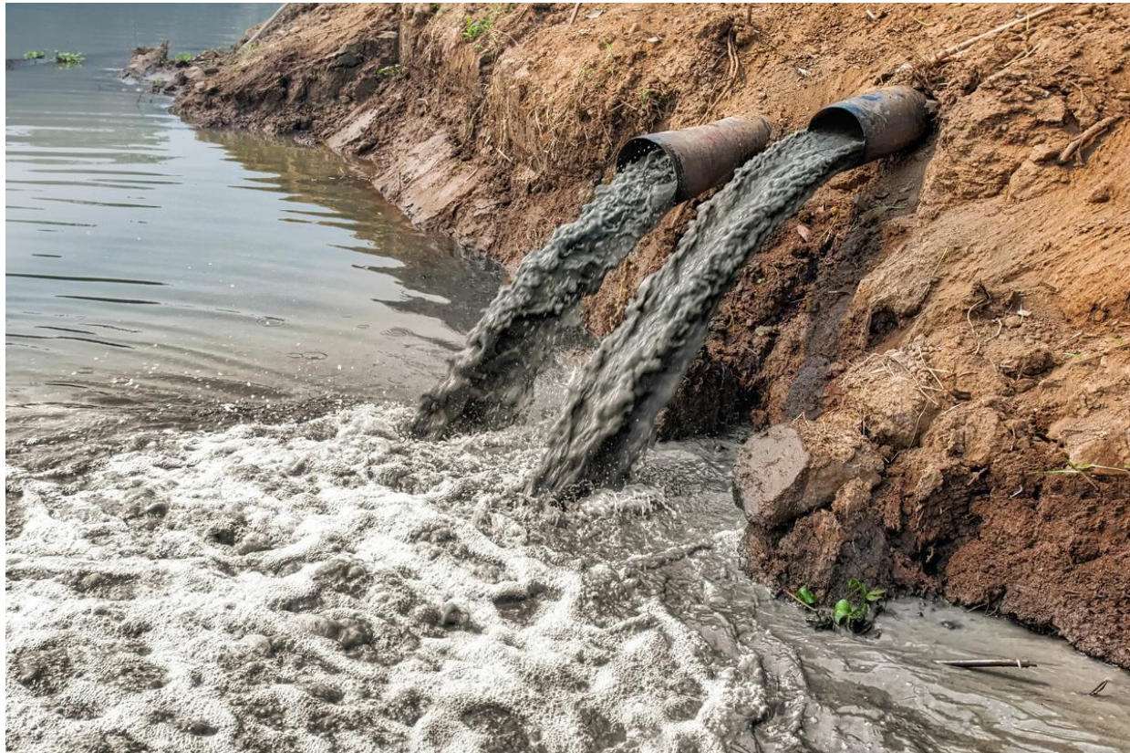
Image No 111: Sewage water discharge, Sankrail Municipality, 22°33'8.06"N 88°18'24.16"E
