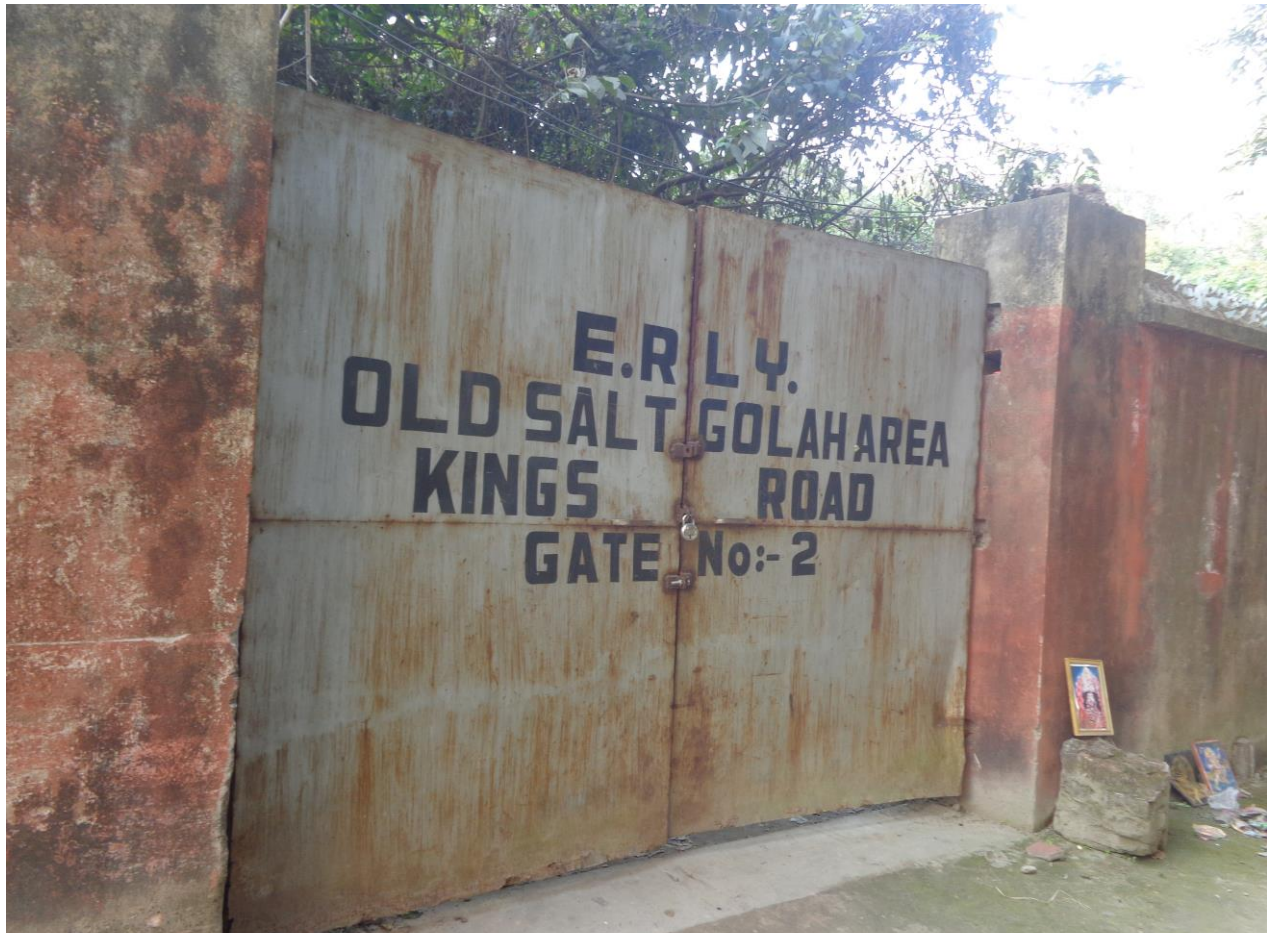
Image No 96: On the western banks of the Hooghly River, seven kilometres west of Calcutta, stands a fiery red brick building. It is the 200-year-old Salt Golah of Howrah — dilapidated, abandoned, a prisoner of aerial roots and creepers.
